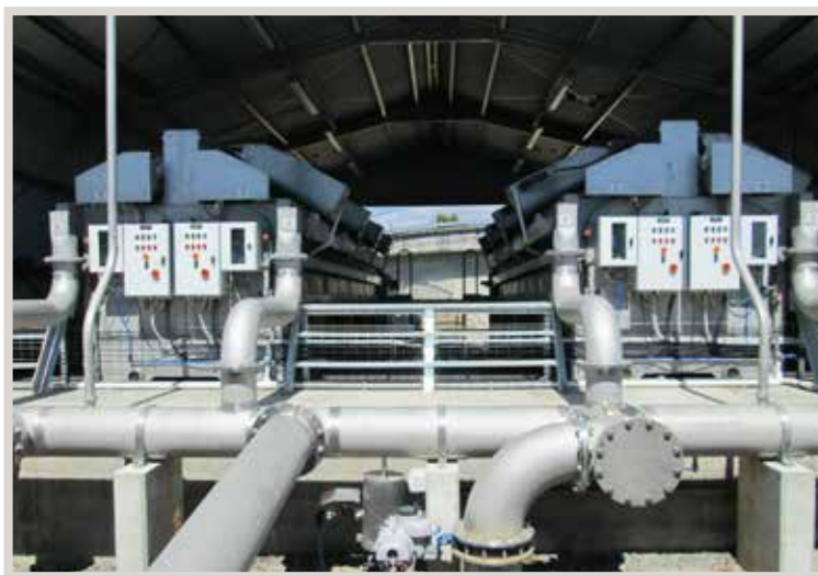
FILTRATION SYSTEM - TE KUITI WASTEWATER TREATMENT PLANT
